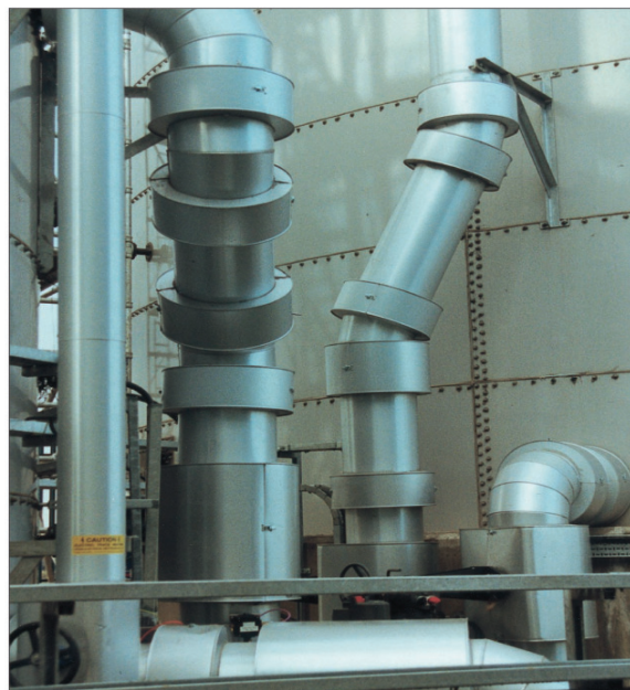
Trace Heating and Insulation in Corrosive Environment
